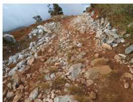
Hurricane Damaged Road
